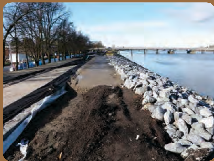
2011 Upgrade to Dike in Fraser River Estuary, Richmond, B.C. (Photo: City of Richmond)
