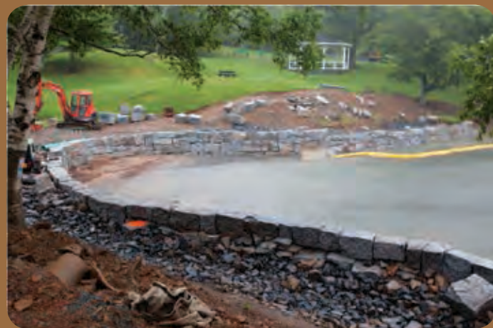
NW Arm Sea wall at Fleming Park under construction June 2012, Halifax, NS
